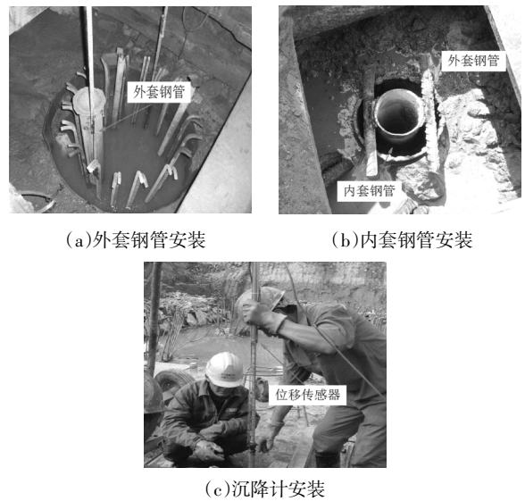
图4 桩底沉降计埋设过程 Fig.4 Installation procedures of settlement gauges below the pile bottom
