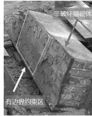
图7 未明显破坏区域的砌体 Fig. 7 Not obviously damaged area of masonry
